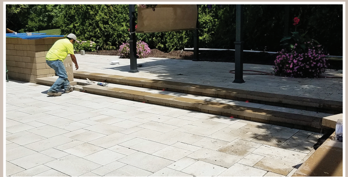
Routing wires under and behind the hardscape helps to reduce damage to wire and eliminate unsightly wires.
